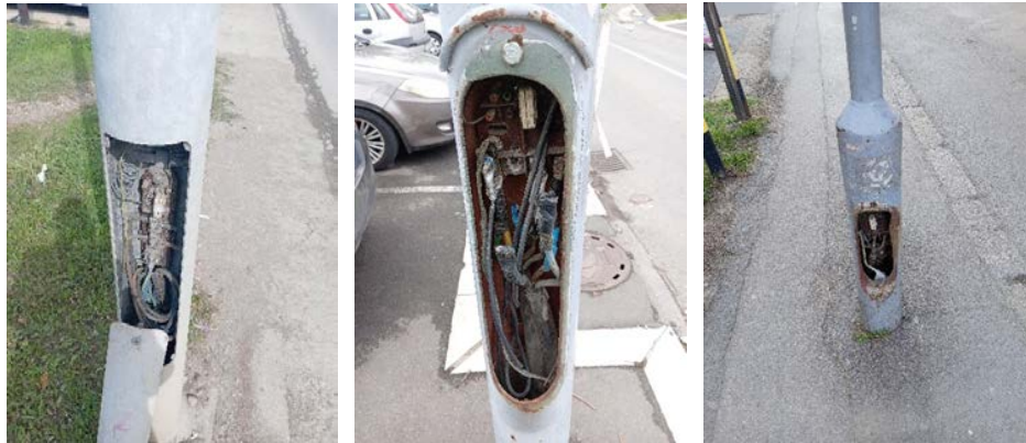
Figure 2. Removed covers on street-lighting poles.
