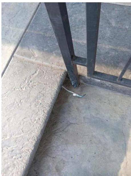
Figure 5. A power cable with uninsulated wires located near the base of a metal fence.
