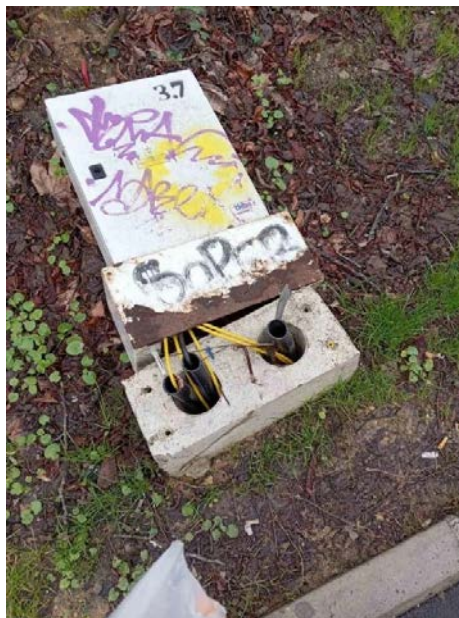
Figure 3. Damaged metal distribution cabinet.
