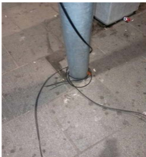
Figure 4. Several cables wrapped around a metal pole.
